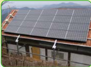
With solar panel
